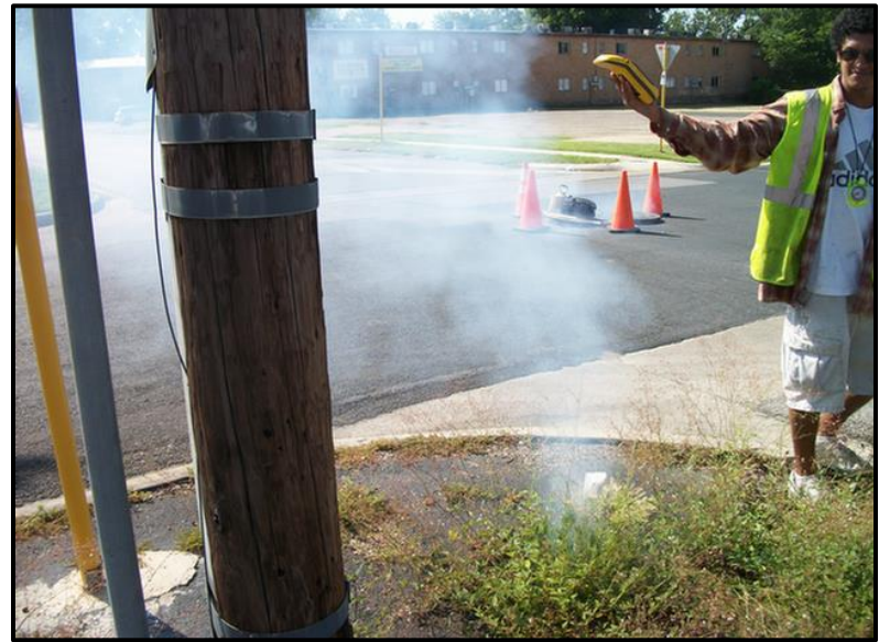
Sewer Line SSES Phase 4
