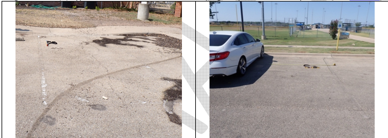
Figure 3.2.1.2(b) Typical Observation: Access aisle striping not provided or badly faded: [TAS 502.3.3. ]
