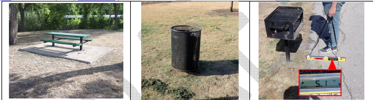
Figure 3.3.1.2(b) Typical Observation: No accessible route to amenities such as picnic tables and grills. [TAS 206.2.2 and ABAAS (ODA) F245.2.5.1. ]
