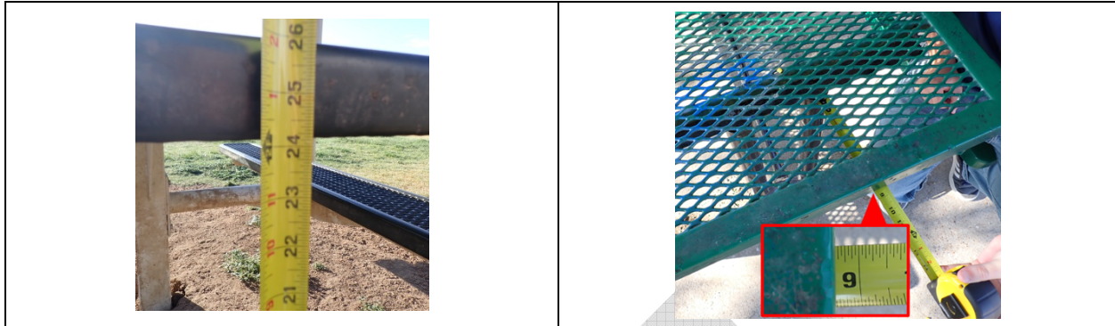
Figure 3.3.1.2(a) Typical Observation: Insufficient knee clearance at picnic table. [TAS 306.3.3. ]
