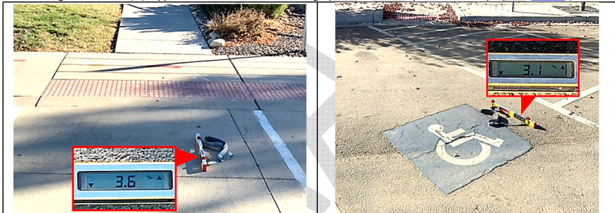
Figure 3.2.1.3(b) Typical Observation: Parking spaces with slopes too steep: [TAS 502.4 .]
