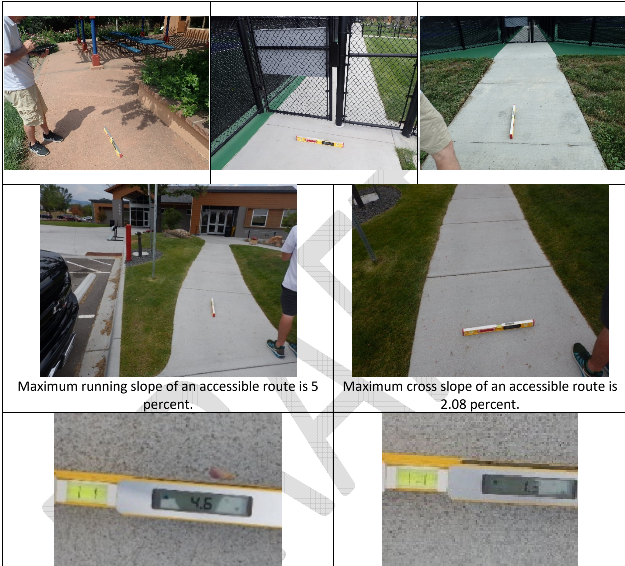
Figure 3.2.1.3(d) Typical Observation: Accessible routes with slopes too steep: [TAS 403.3 ]
