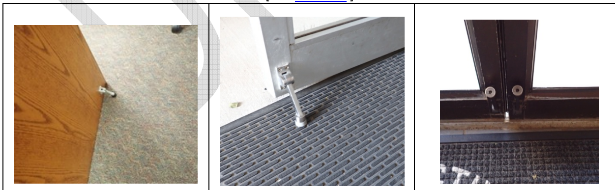
Figure 3.2.1.1(e) Typical Observation: 10-inch smooth surface missing on the push side of doors: [TAS 404.2.10. ]
