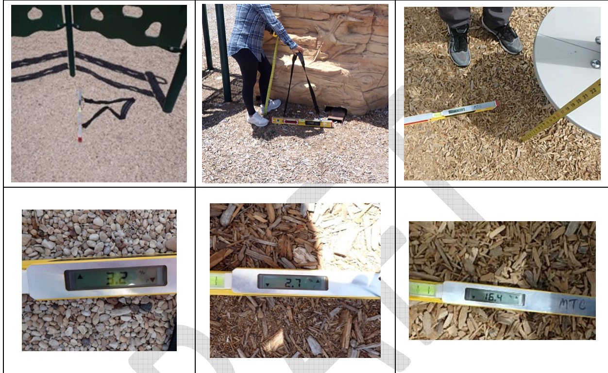
Figure 3.3.1.3(a) Typical Observation: Maximum slope of the clear space at play area ground component is steeper than 2.0 percent. [ADA Standards 1008.4.2 , and 305.2 ]
