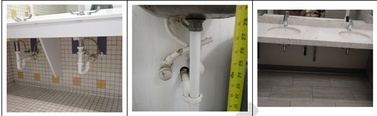
Figure 3.2.1.1(g) Typical Observation: Water supply and drain lines are not insulated under lavatories: [TAS 606.5. ]
