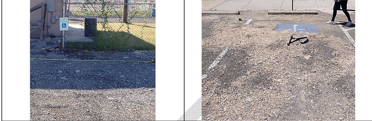
Figure 3.2.1.3(a) Typical Observation: Surface not firm and stable: [TAS 302 referenced from 502.4 ]
