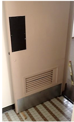
Door with smooth push side surface within 10 inches of finish floor.
