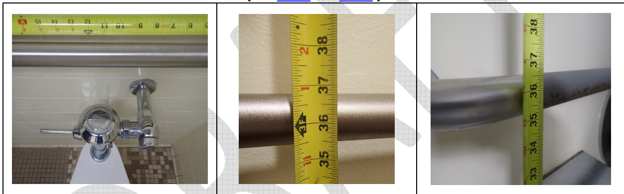
Figure 3.2.1.1(f) Typical Observation: improperly mounted grab bars in restrooms: [TAS 604.5 and 609.4 .]
