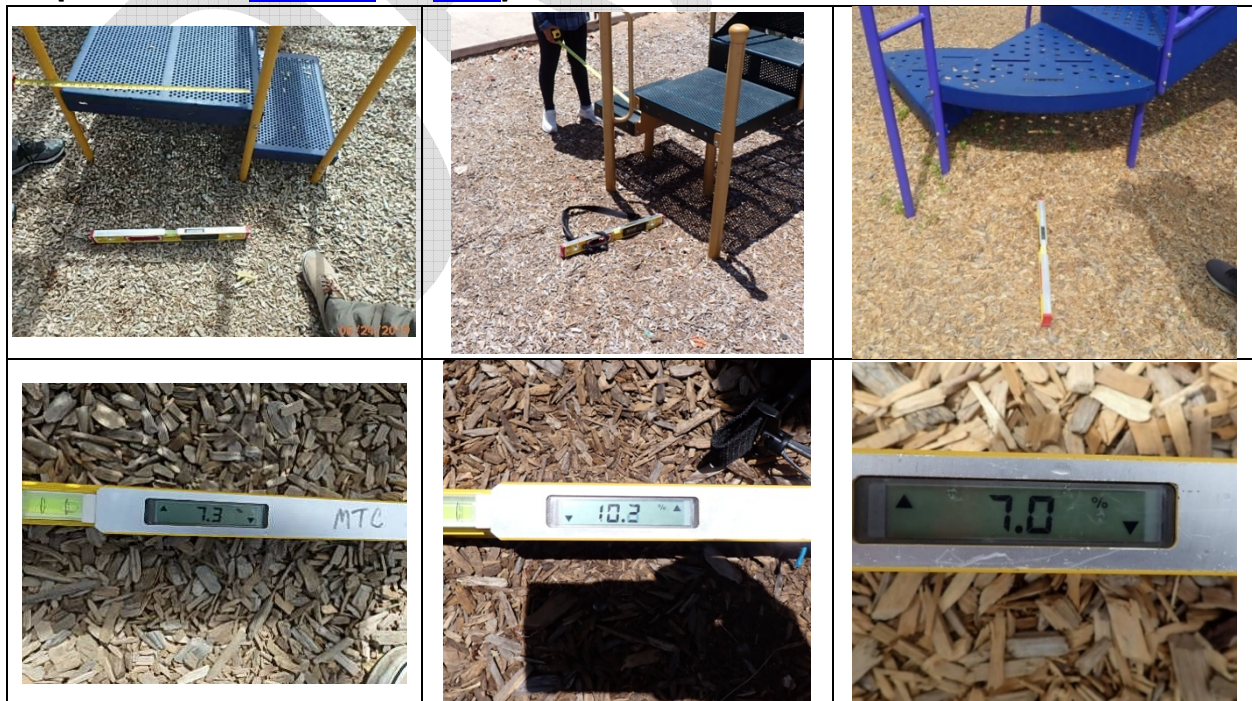
Figure 3.3.1.3(b) Typical Observation: Maximum slope of the transfer space at play area transfer platform is 2.1 percent. [ADA Standards 1008.3.1.3 and 305.2 ]
