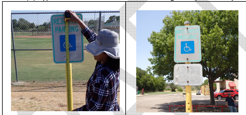
Figure 3.2.1.1(d) Typical Observation: Van accessible sign not provided: [TAS 502.6. ]
