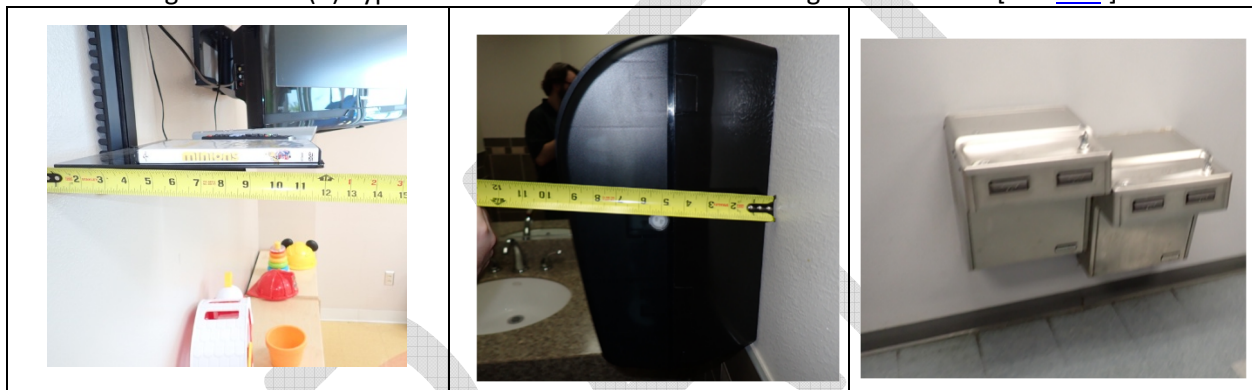
Figure 3.2.1.1(b) Typical Observation: Protrusions throughout facilities: [TAS 307. ]
