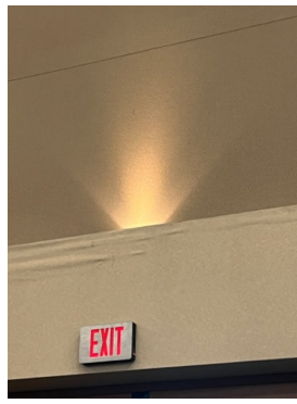
Example of light that need to be protected
