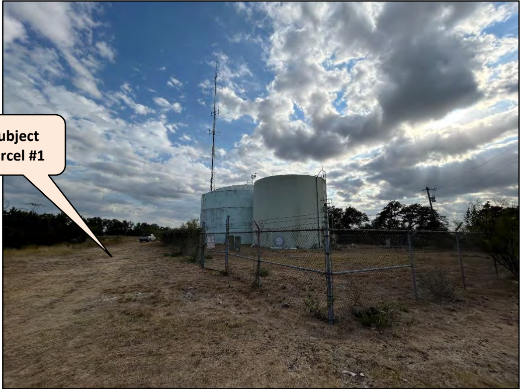
Existing Two Water Tanks, which will be demolished and replaced with two new larger water tanks
